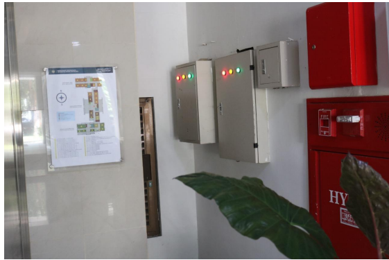
Mesin Panel Listrik Genset
